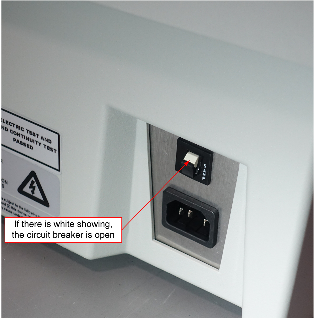
Figure 4-19: Open circuit breaker
